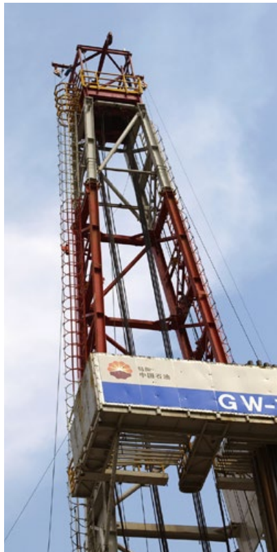
Drilling in Rwanda. Iceland and the Nordic Development Fund participate in geothermal projects in East Africa
